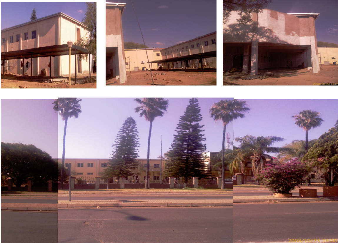
Photos 15 – 19: The side views (3) and front view (1) of the Main Municipal Building during construction which was said to be completed during 2008/ 09 financial year.
